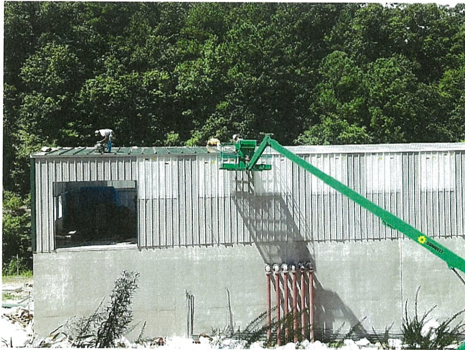
Construction progress of SDCRWA WTP. Sheet Metal has finally arrived and is going up.
