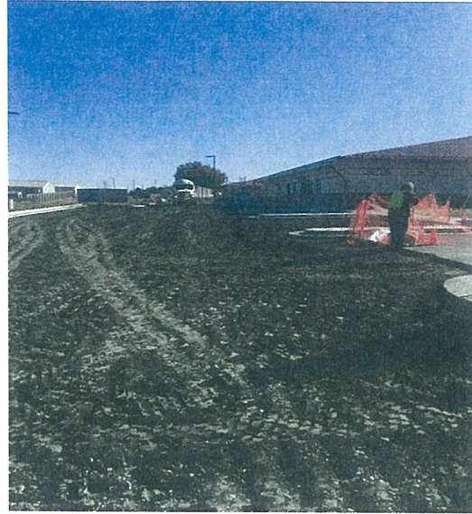
Redbird Clinic pavement
